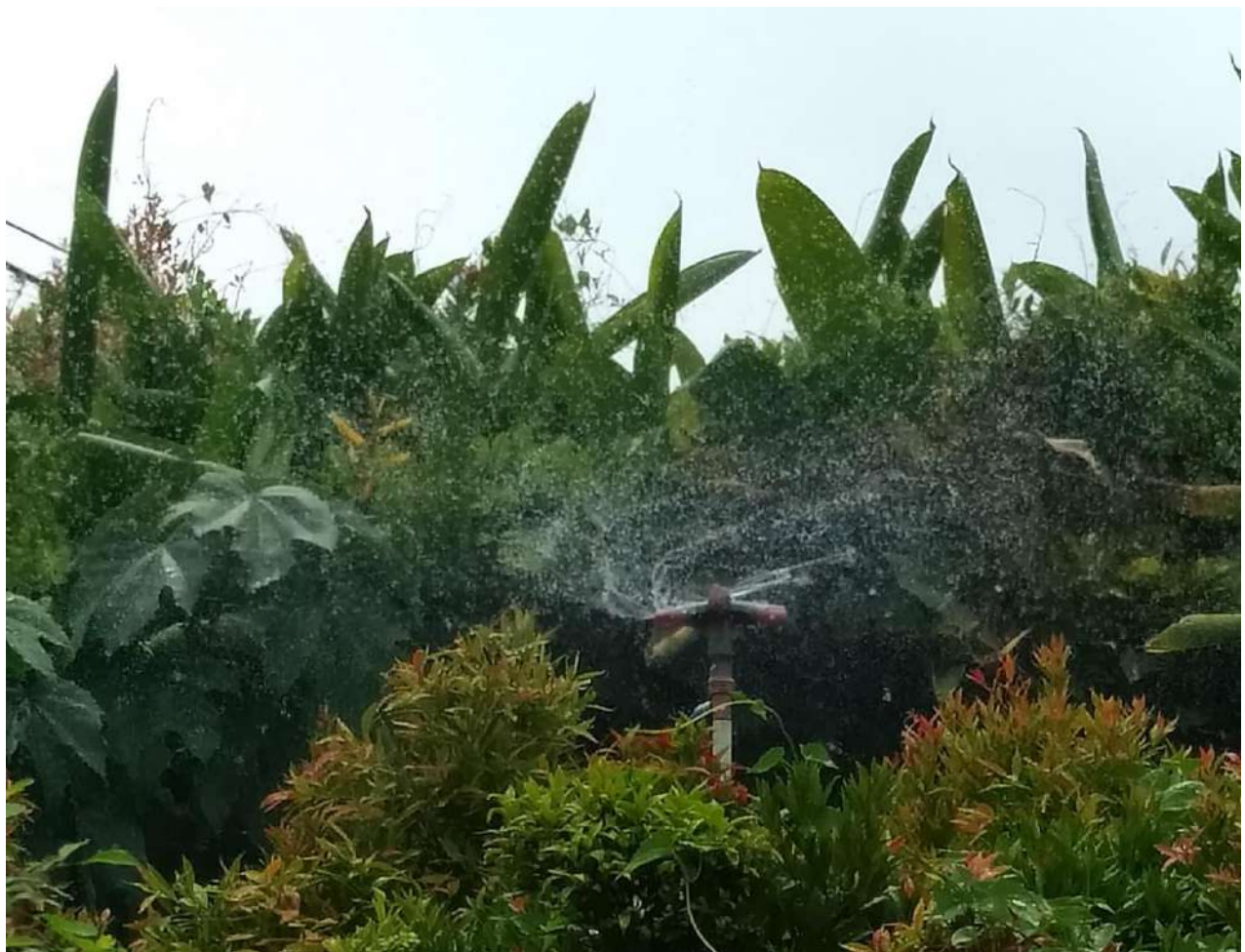
Use of water-saving fixtures
