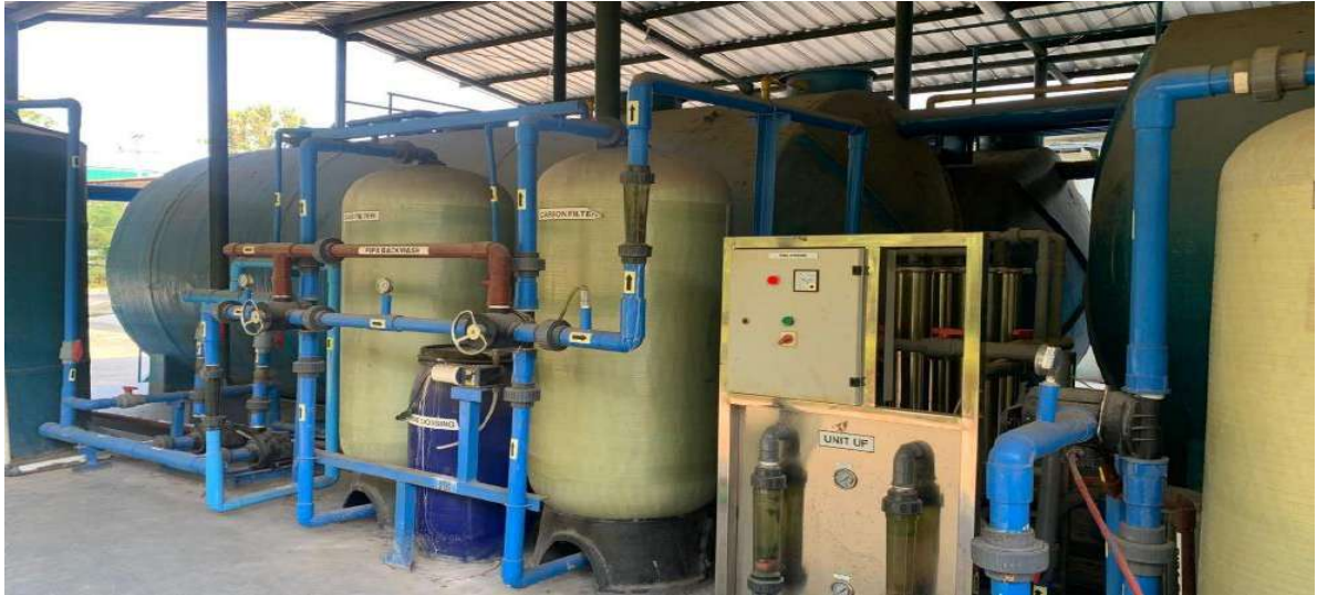
WWTP from Processing in Bio Filter
