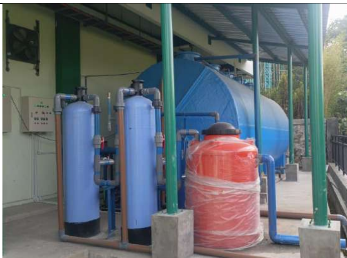
Bio Filter Reservoir on the Floor
