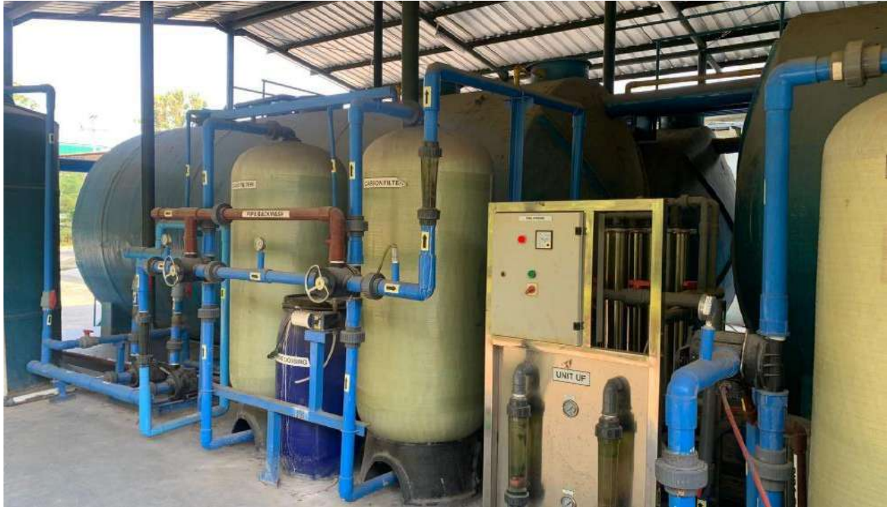
WWTP from Processing in Bio Filter
