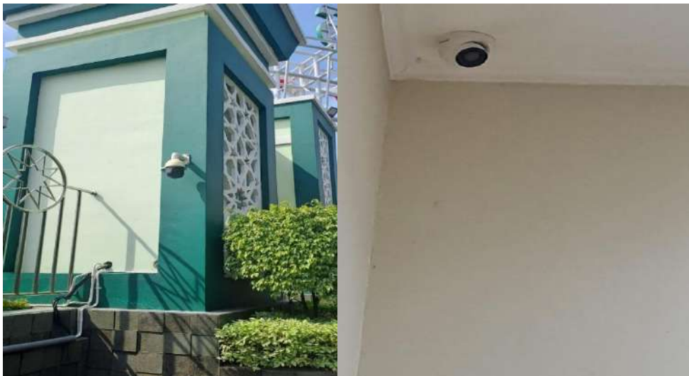
CCTV environment and in the building
