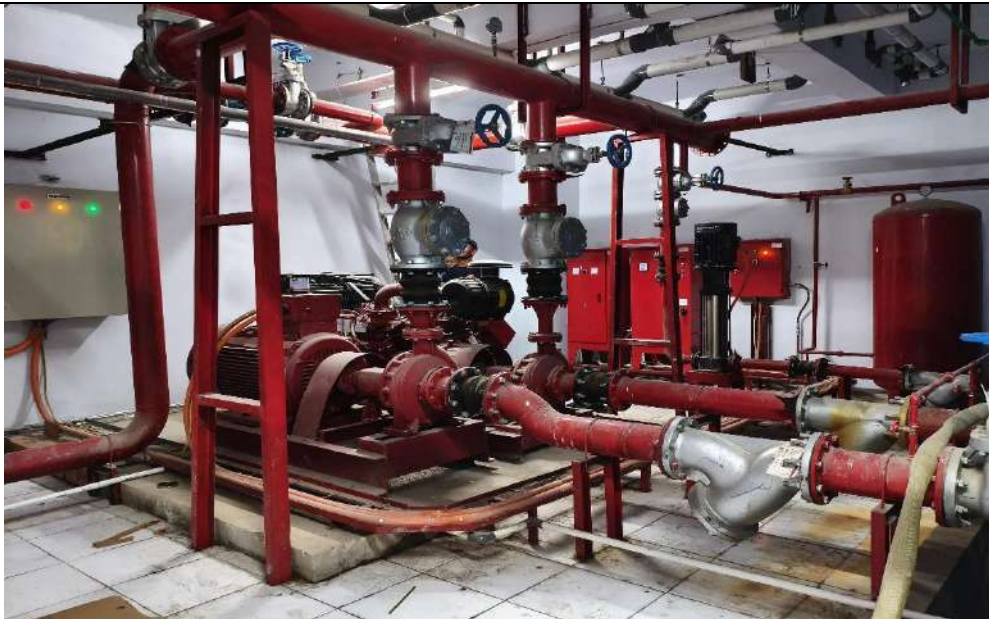
Hydrant Pump and Springler System
